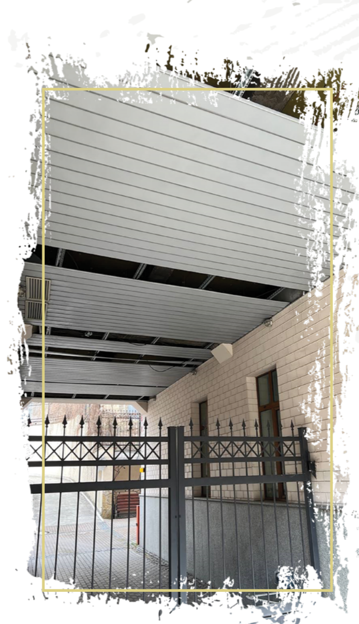
Picture 2.3. The SFMS building facade damaged by the blast wave from a Russian missile, March 15, 2022
